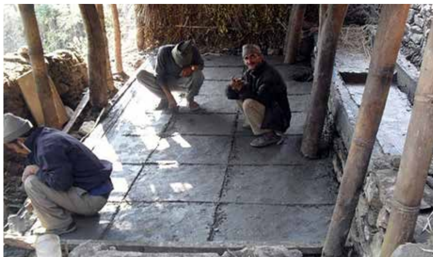
Cattle shed improvement through construction of new sloping floor, feeding manger and urine collection tank, Ramechhap, 2012
