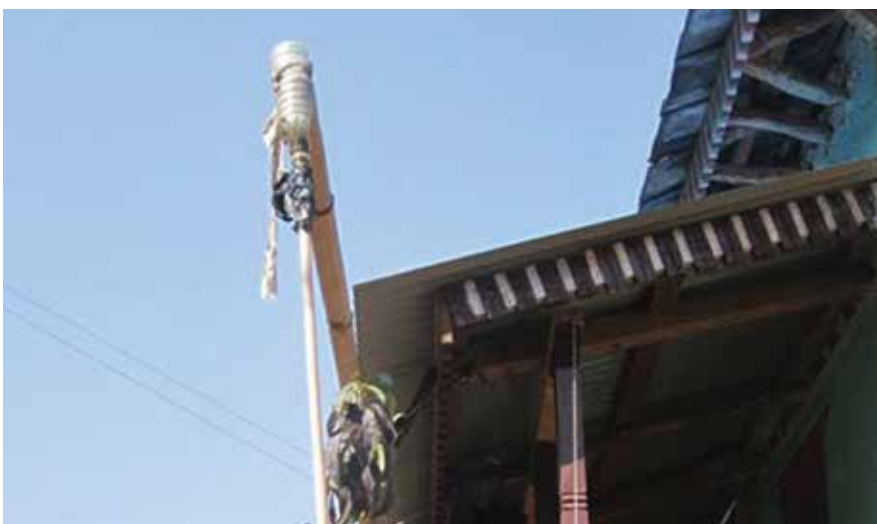
A bamboo gutter collecting rain from zinc sheet roofing, Okhaldhunga, 2013
